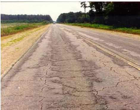
Figure 4.1: Typical reflective cracking from a CTB pavement
