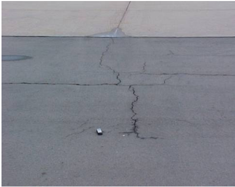
Figure 4.2: Cracking adjacent to concrete pavement
